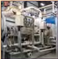
8 Cogeneration Facilities We turn wood waste into energy to run our mills
